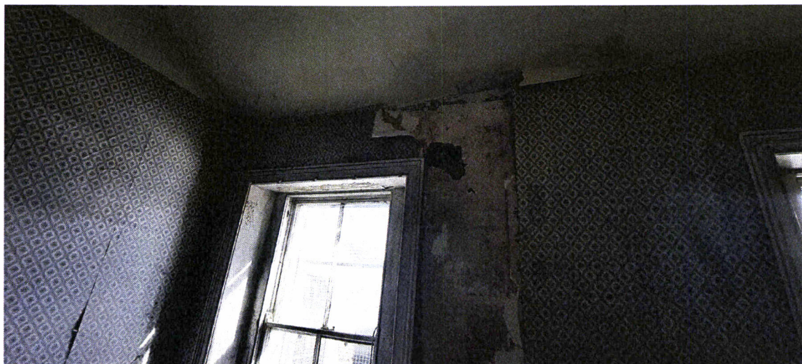
Interior corner, multi-layer wallpaper, wired safety glazing window with external roofline view, plaster damage at wall-ceiling junction
