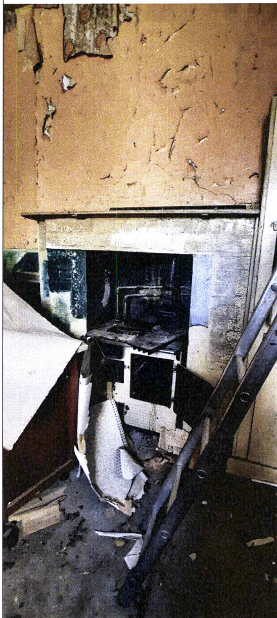
Interior, redundant cast-iron solid fuel range and masonry surround, severe distemper deterioration and damp staining to wall above 2026-04-01.
